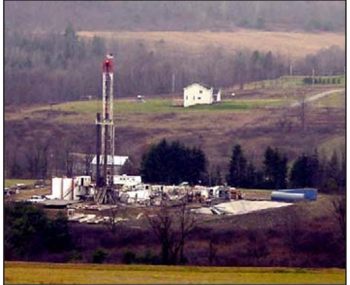
Drilling a Trenton Black River well at the edge of a suburban community.
